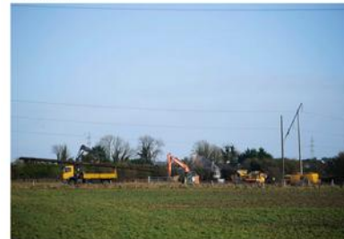
Crews from ESB Networks replace fallen electricity poles in a field near Galway Airport after they were damaged during Storm Isha. Photograph: Neil Carson/RTÉ News
